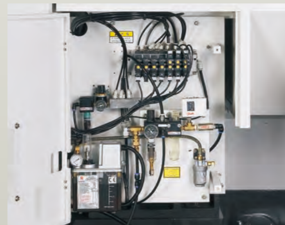
Hydraulic & Lubrication System(LU-620)
